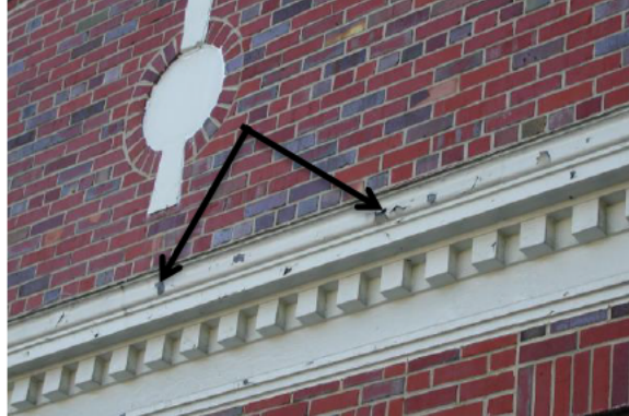
Unpainted Molding on Building Front
